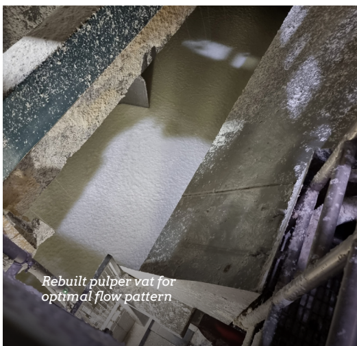
SCV Expansion 2.0 / Broke Handling
